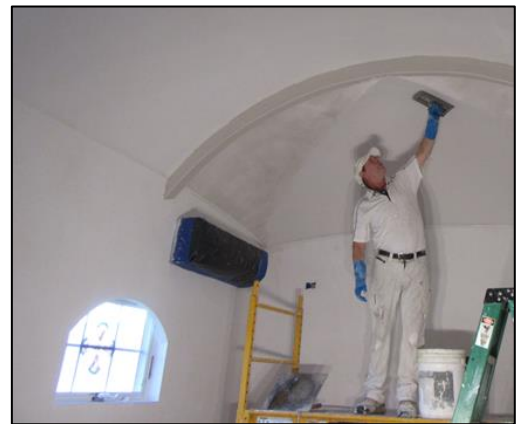
The Skete was blessed to have the chapel walls, ceiling and vaults finished by master craftsman Paul King, a British native who learned the art of plastering in the Old-World style – made to last for generations.
